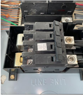
Main breaker panel - Up close
