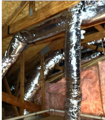
Flexible HVAC ductwork in attic
