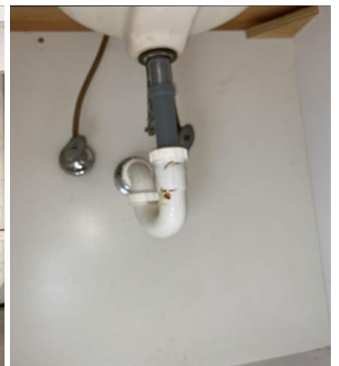
Single supply line under sink with p-trap
