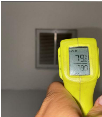
Return air temperature
