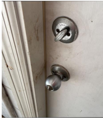
Lock was damaged.
