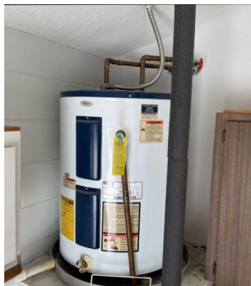
Residential electric water heater installation
