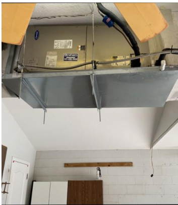
Air handler unit in garage ceiling
