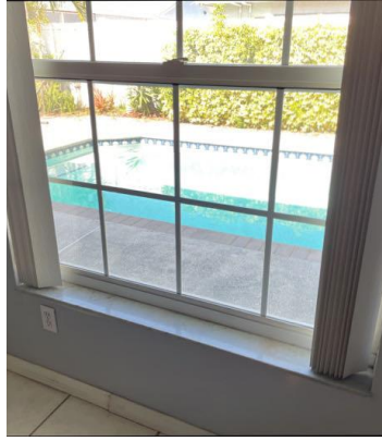
Window tension spring(s) were damaged - Utility room
