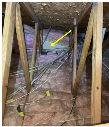
Electrical box exposed in attic insulation
