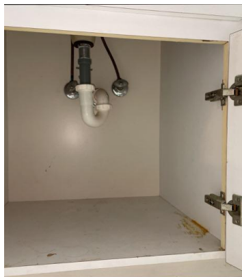
Bathroom sink plumbing under cabinet
