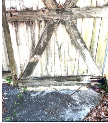
Gate was damaged
