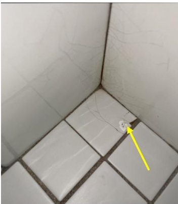
Cracked tiles were visible at primary bathroom
