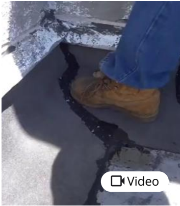
Roof water damage
