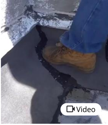
Roof water damage
