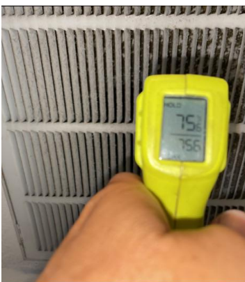
Return air temperature
