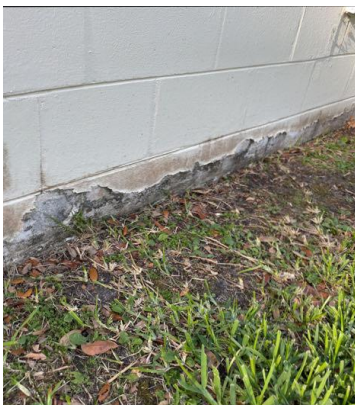
Paint is peeling at the ground
