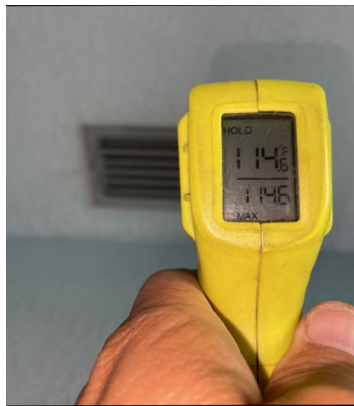
Supply air temperature
