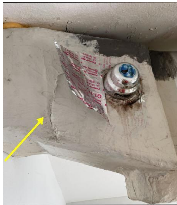
Gaps/damage at the plenum should be sealed.
