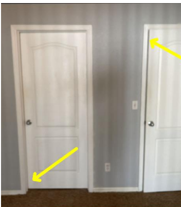
Door rubbed/stuck at primary bedroom
