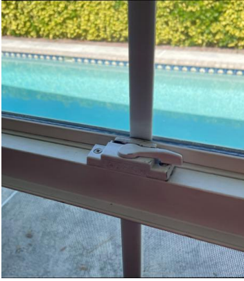
Locks were missing/damaged at family room
