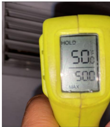
Supply air temperature
