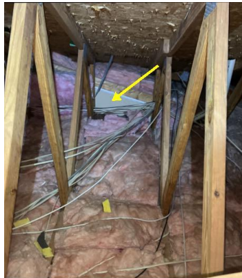
Electrical box exposed in attic insulation
