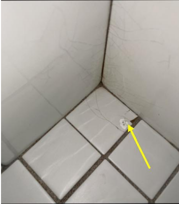
Cracked tiles were visible at primary bathroom
