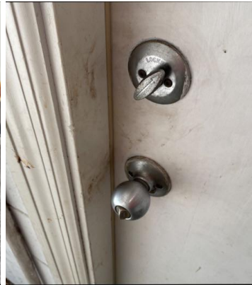
Lock was damaged.
