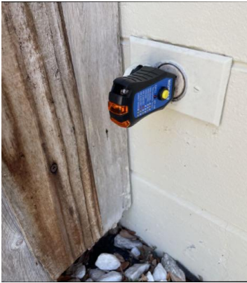
Outlet(s) were not operational at exterior.
