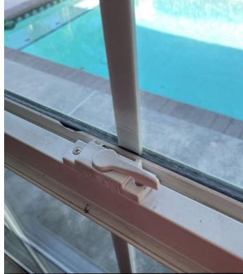
Locks were missing/damaged at family room
