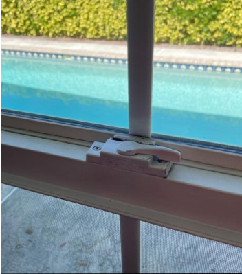
Locks were missing/damaged at family room
