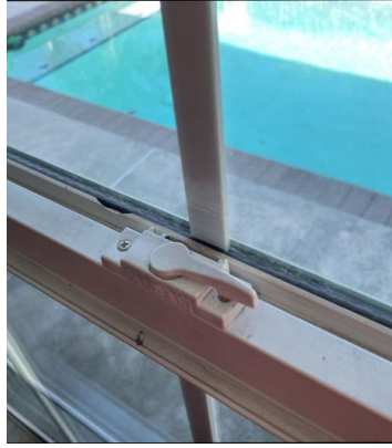
Locks were missing/damaged at family room
