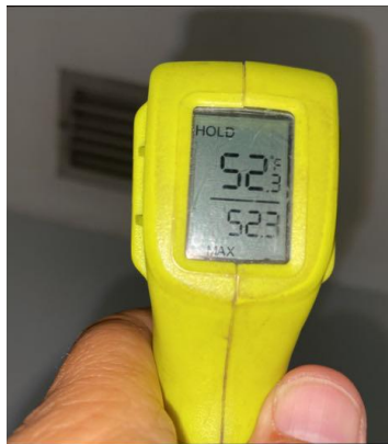
Supply air temperature
