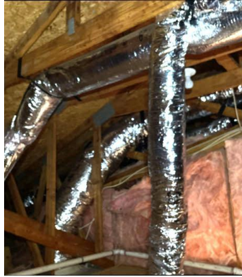
Flexible HVAC ductwork in attic
