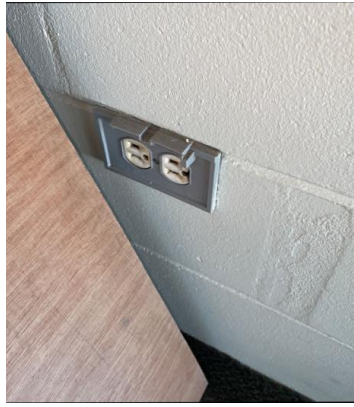
Weatherproof covers were damaged/missing at exterior outlet(s).
