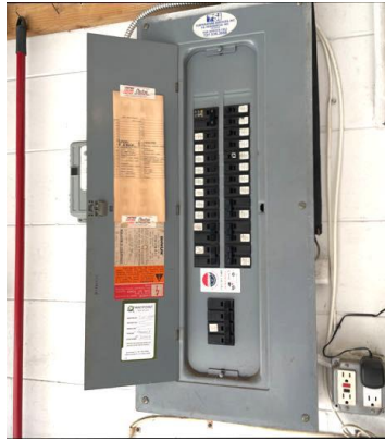
Electrical panel - Open
