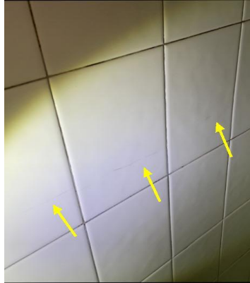
Cracked tiles were visible at primary bathroom
