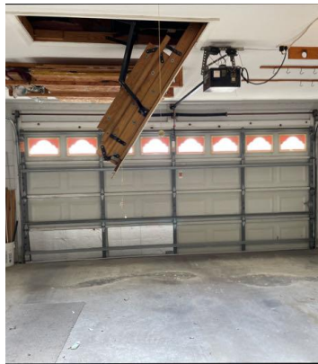
Garage door - Closed
