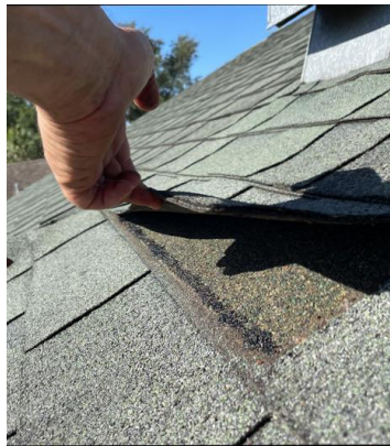
Loose shingles near vent flashing
