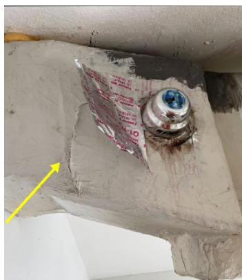
Gaps/damage at the plenum should be sealed.
