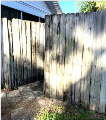
Fence was damaged.
