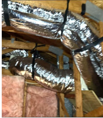
Flexible HVAC ductwork in attic
