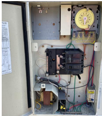
Outdoor electrical sub-panel - Open
