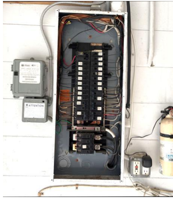
Electrical panel - Door off
