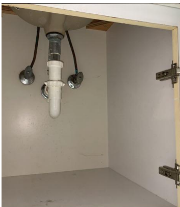
Bathroom sink plumbing under cabinet
