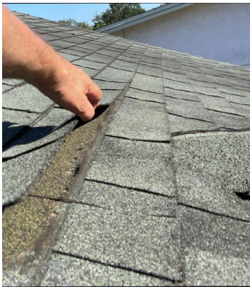
Lifted roof shingles at ridge
