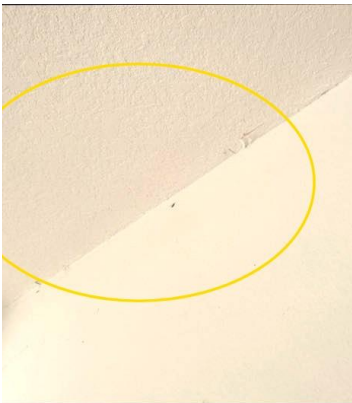
Ceiling seam separation was visible.
