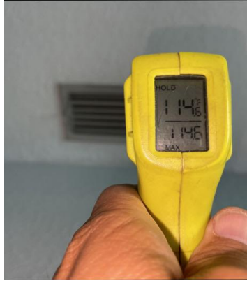
Supply air temperature
