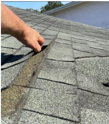
Lifted roof shingles at ridge
