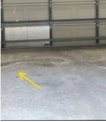
Stainging on garaga floor
