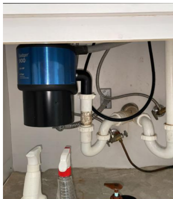
Kitchen sink with garbage disposal
