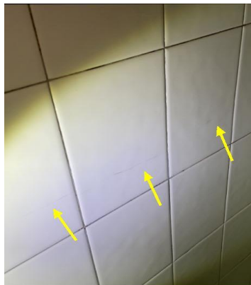
Cracked tiles were visible at primary bathroom
