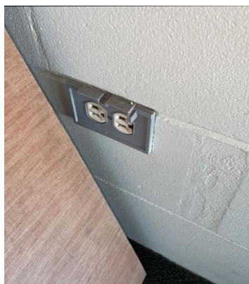
Weatherproof covers were damaged/missing at exterior outlet(s).
