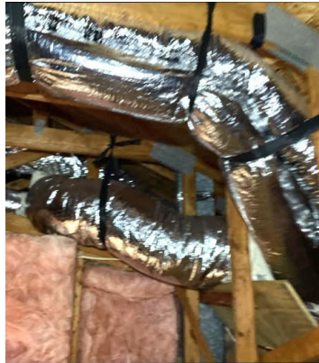
Flexible HVAC ductwork in attic
