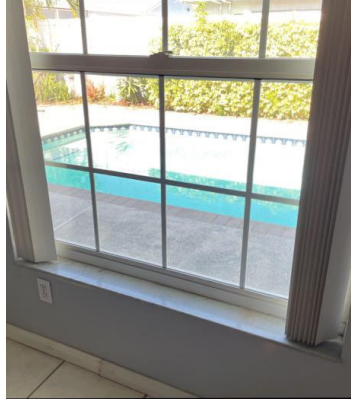
Window tension spring(s) were damaged - Utility room
