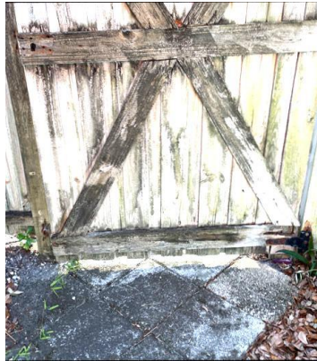
Gate was damaged
