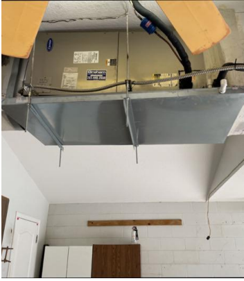
Air handler unit in garage ceiling
