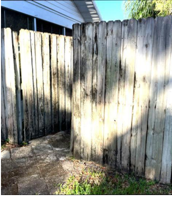
Fence was damaged.
