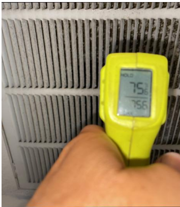
Return air temperature
