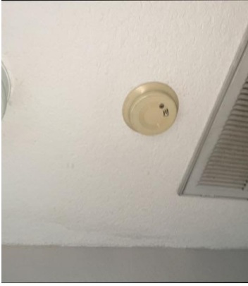
Smoke detector(s) did not respond when tested at Hallway
